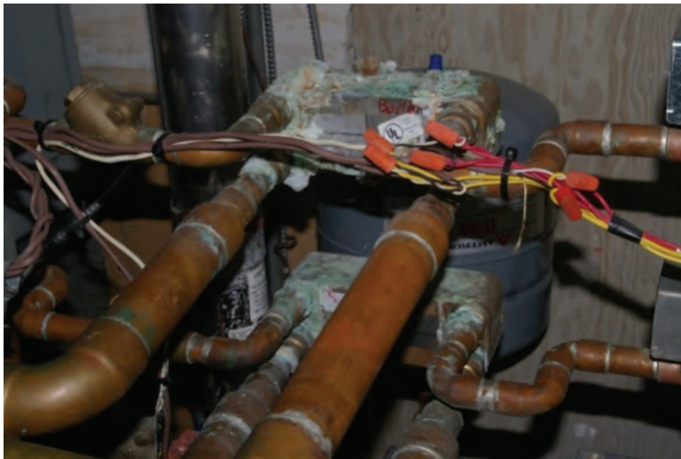
Photo 2.1.5 Detail showing heat exchangers used with domestic water system approximately 12 years old. Note the build up of deposits on the heat exchangers.
