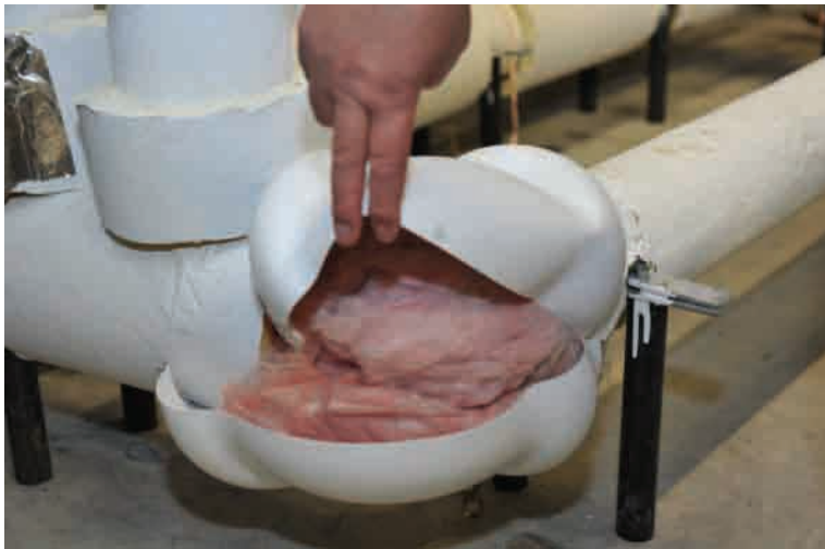
An example of an improper system with no vapour barrier and use of pink insulation instead of a matched density flexible insulation equivalent to the adjacent pipe covering.
