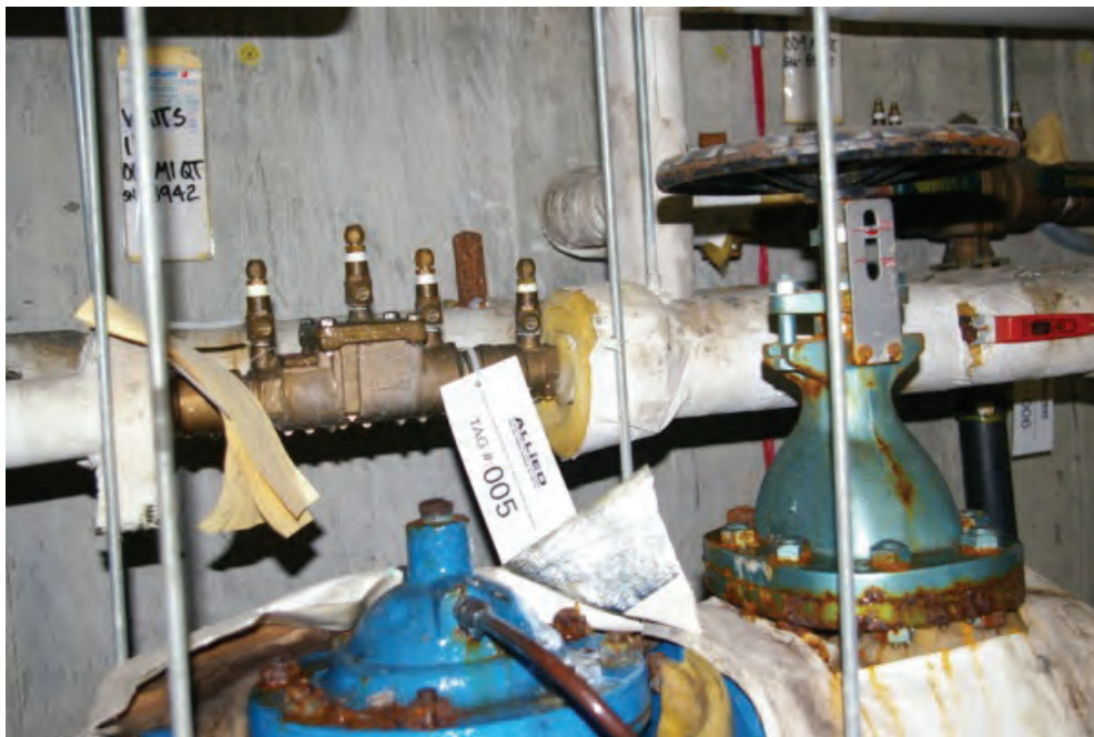
Photo 2.1.3 Detail showing backflow preventer on domestic water supply line. Note the water dripping from the device.
