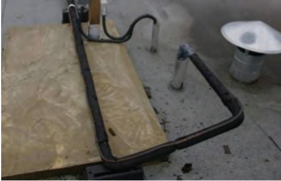
Photo 2.1.6 Detail showing rubber insulation on a hot gas refrigerant line. The insulation should be jacketed to protect it from sun and birds.
