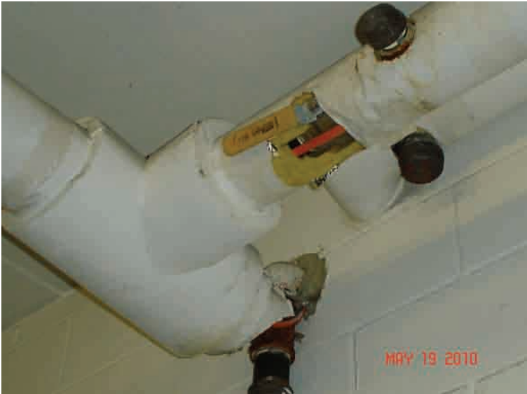
Incomplete and damaged insulation in underground parking of a retailer.
