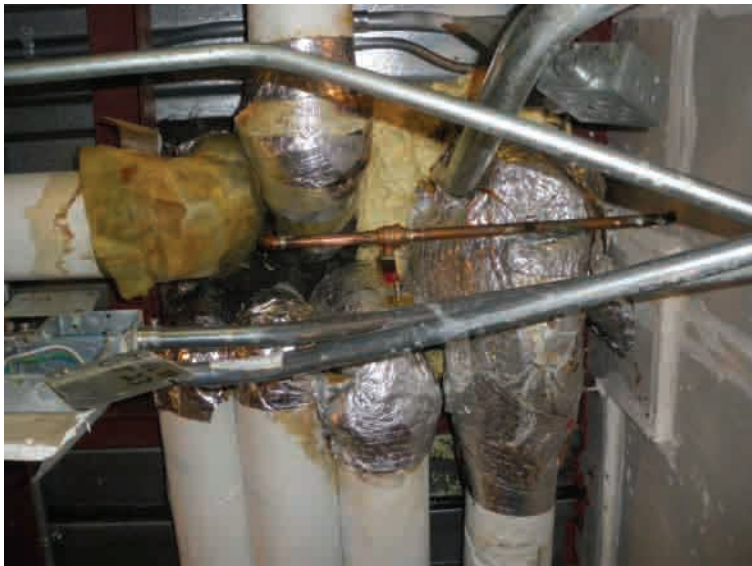
Sweating pipes in a medical building in Vancouver. Note insufficient space adds to the problem.
