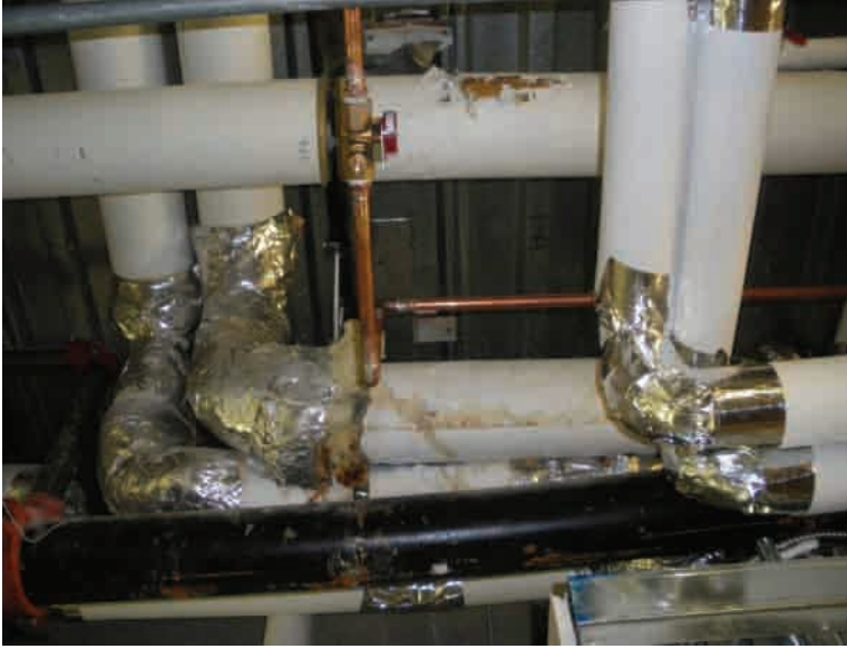
Further evidence of sweating and corrosion at a medical facility. Note that even though the insulation appears to be sealed along the longitudinal seam, the poor quality insulation vapour barrier is not performing as it is supposed to.
