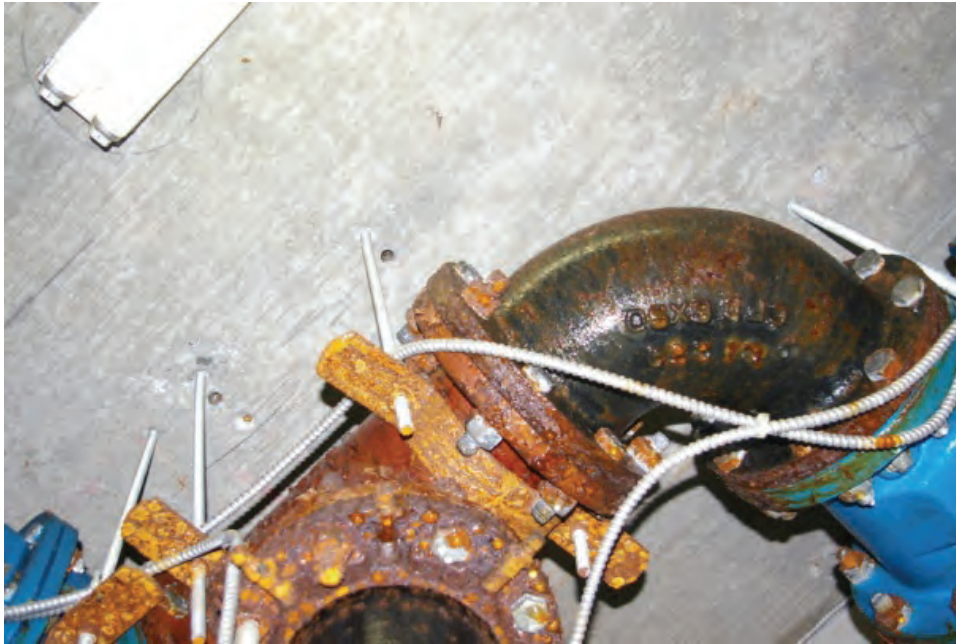
Photo 2.1.4 Detail showing corrosion damage to pipe fittings as the result of condensation.
