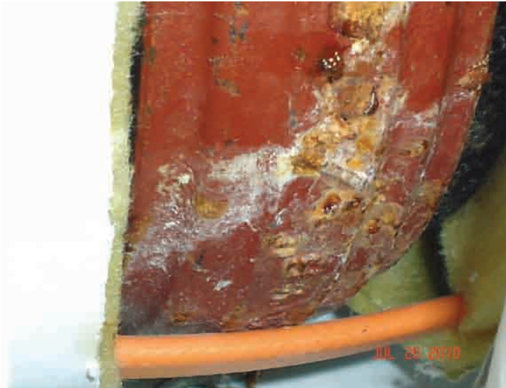
Corrosion and condensation in new Vancouver condominiums
