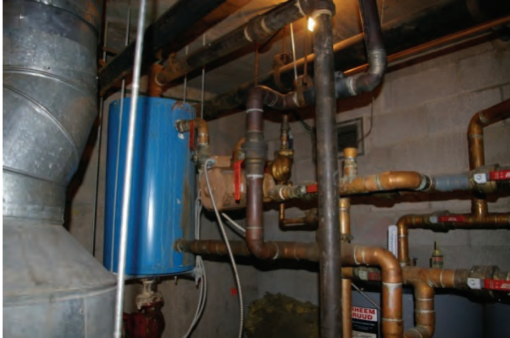
Photo 2.1.2 Detail showing un-insulated hydronic distribution system and heat exchanger for domestic hot water system
