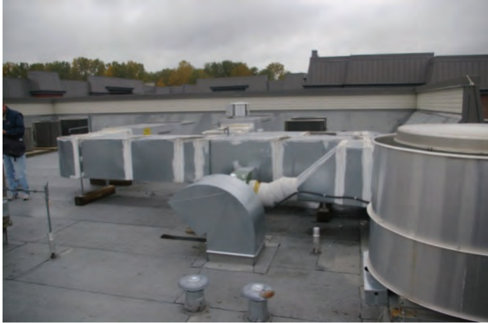
Photo 2.1.7 Detail showing a section of an un-insulated supply air duct on a roof mounted make-up air unit.
