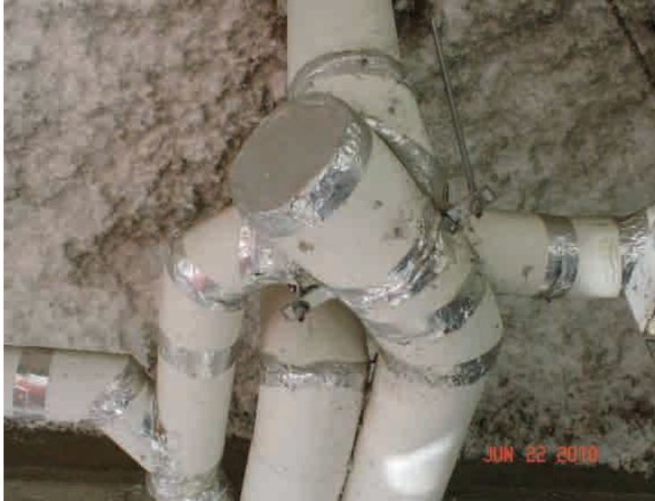
Poorly finished pipe covering in an outdoor parkade. No weather proof jacketing or elbows.
